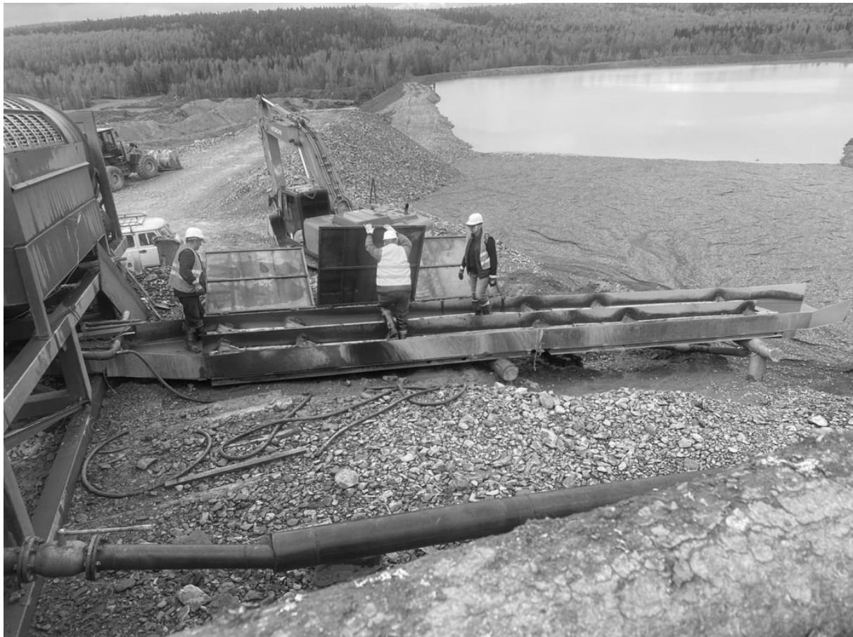
People working on one of the six treatment plants at West Kytlim. Source: Company
